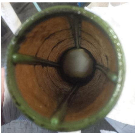
Figure 5: Precipitated wax on strainer element used in the quench fluid circulation system
